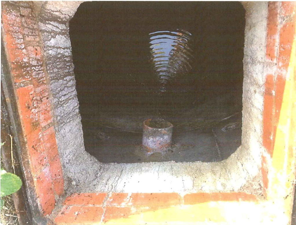
View inside soakaway. Approximately 1800mm diameter concrete rings approximately 1.5m from back of wall. Depth approximately 1.8m
