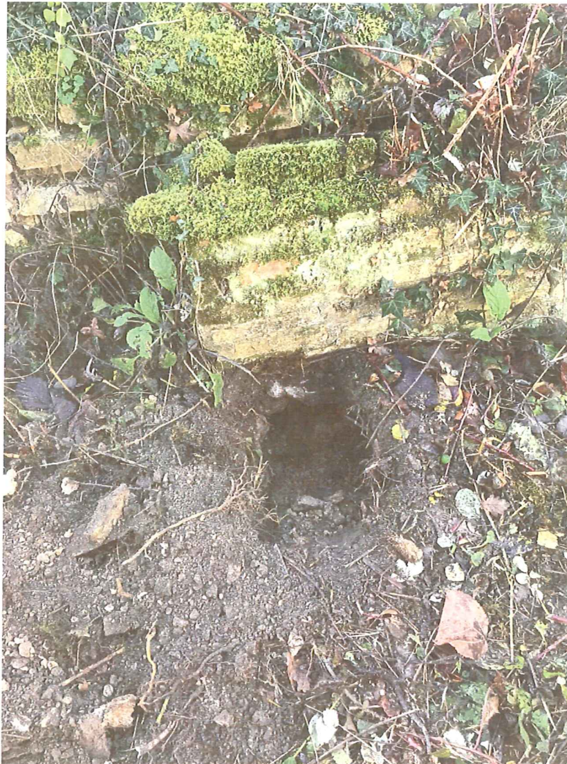
Trial hole within church yard showing upper brickwork capping having shallow foundation with flintwork to main wall set back and extending downwards.
